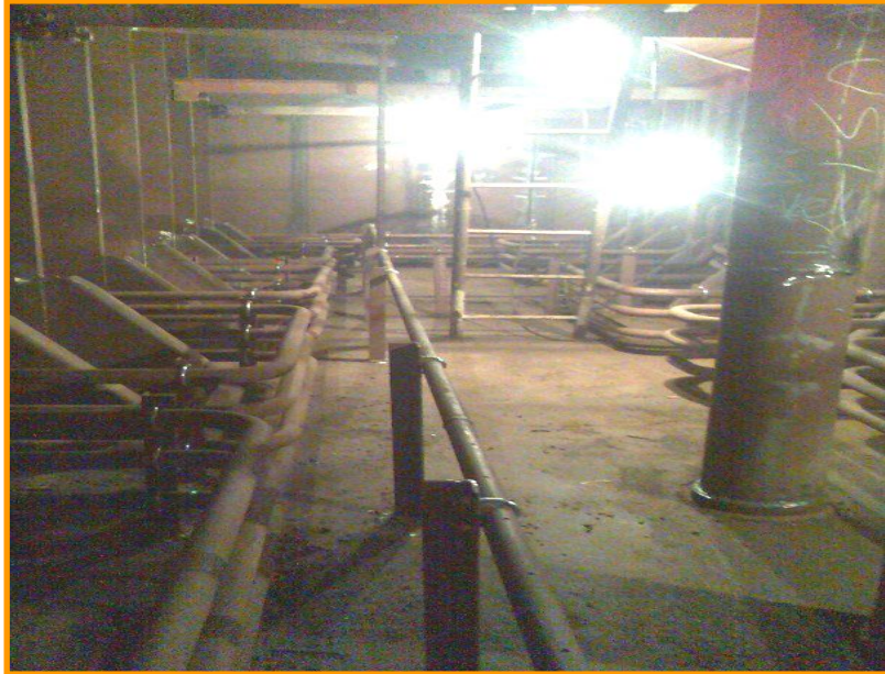
Picture 13. Steam heating coils
