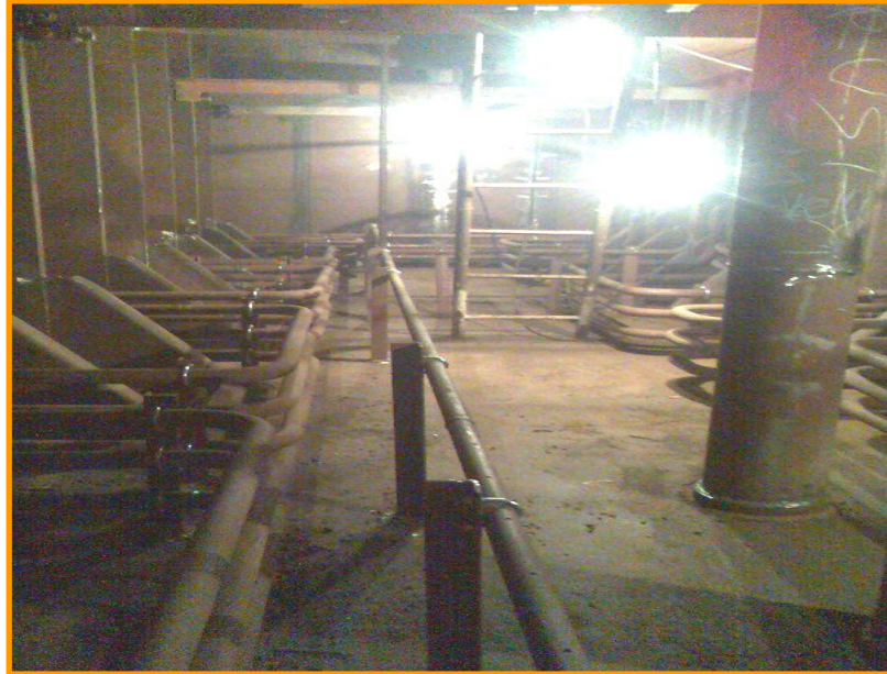
Picture 13. Steam heating coils
