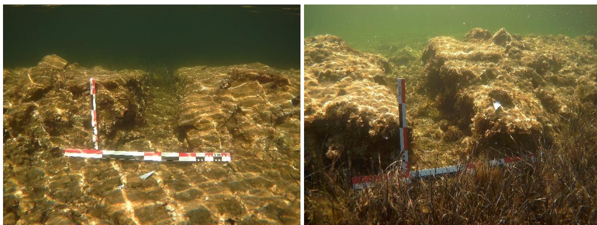
Fig. 108 Sluice gate in the separation wall seen from the internal (a) and from the external (b) part of the wall (M. Grisonic).
