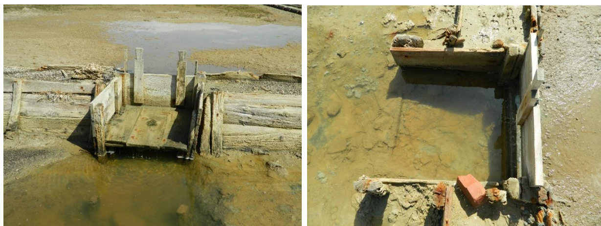
Fig. 58 Sluice gates in between the salt evaporation pools on the saltpans of Pag (M. Grisonic).
