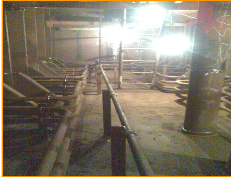
Picture 13. Steam heating coils
