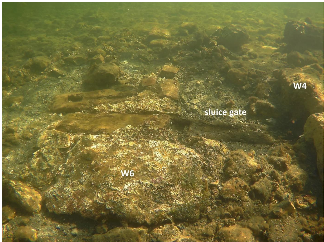
Fig. 113 Probable Wall 6 foundations and a sluice gate in between W6 and W4 (M. Grisonic).
