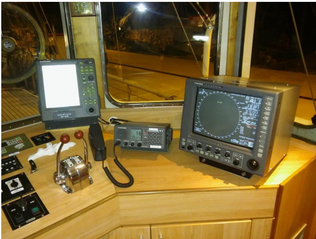
Picture 6. RADAR – Kraljica Mora
